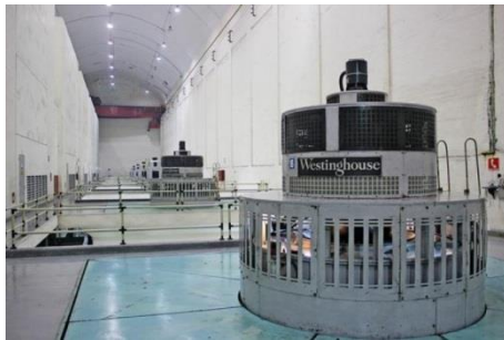
a) Internal View – Generators
