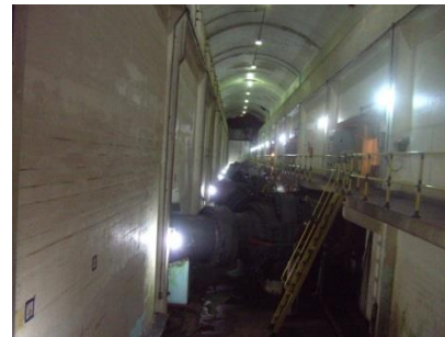
b) Internal View – Valves
